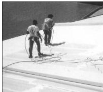
A second finish coat brought the total thickness of the new monolithic rubber membrane to over 30 dry mils on the field and nearly 45 dry mils on all seams, fasteners, curbs and penetrations.
